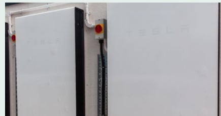
40kW of battery storage
