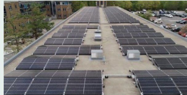
100kW of PV generating 80MWh of electricity per year.
